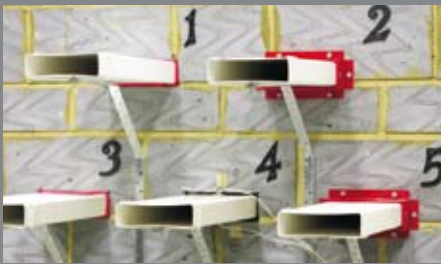
Independent Fire Test: 1. Wrap on one side only, 2. Collar fitted on one side only, 3. Wraps on both sides, 4. The Domus FireBrake centred within the wall, 5. Collars fitted on both sides of the wall.
